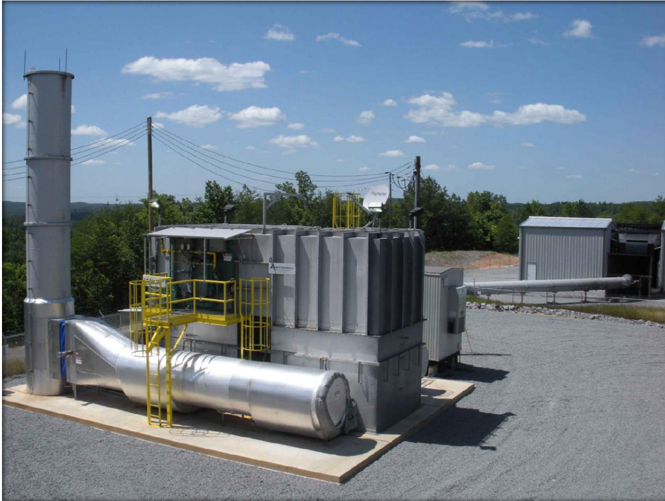
Picture of Biothermica VAMOX ® system (Shows mine shaft, inlet duct and VAMOX ® system)
