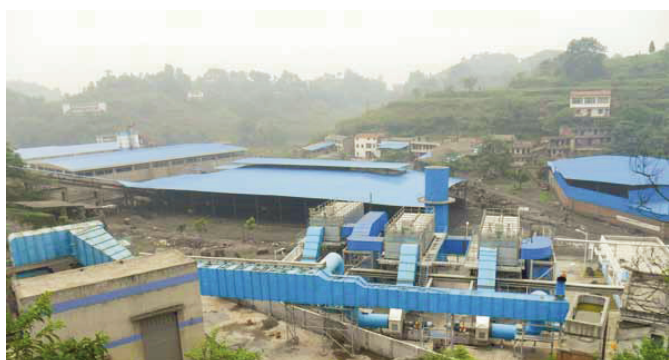
Figure 2. RTO Installation at the DaTong coal mine in Chongqing municipality, China. Image courtesy of MEGTEC.
