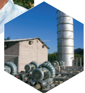
Blowers at the flare ▶
