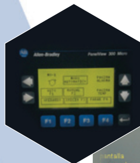
Control panel for flares and collecting system, operated and maintained by Mario Lemus ▶
